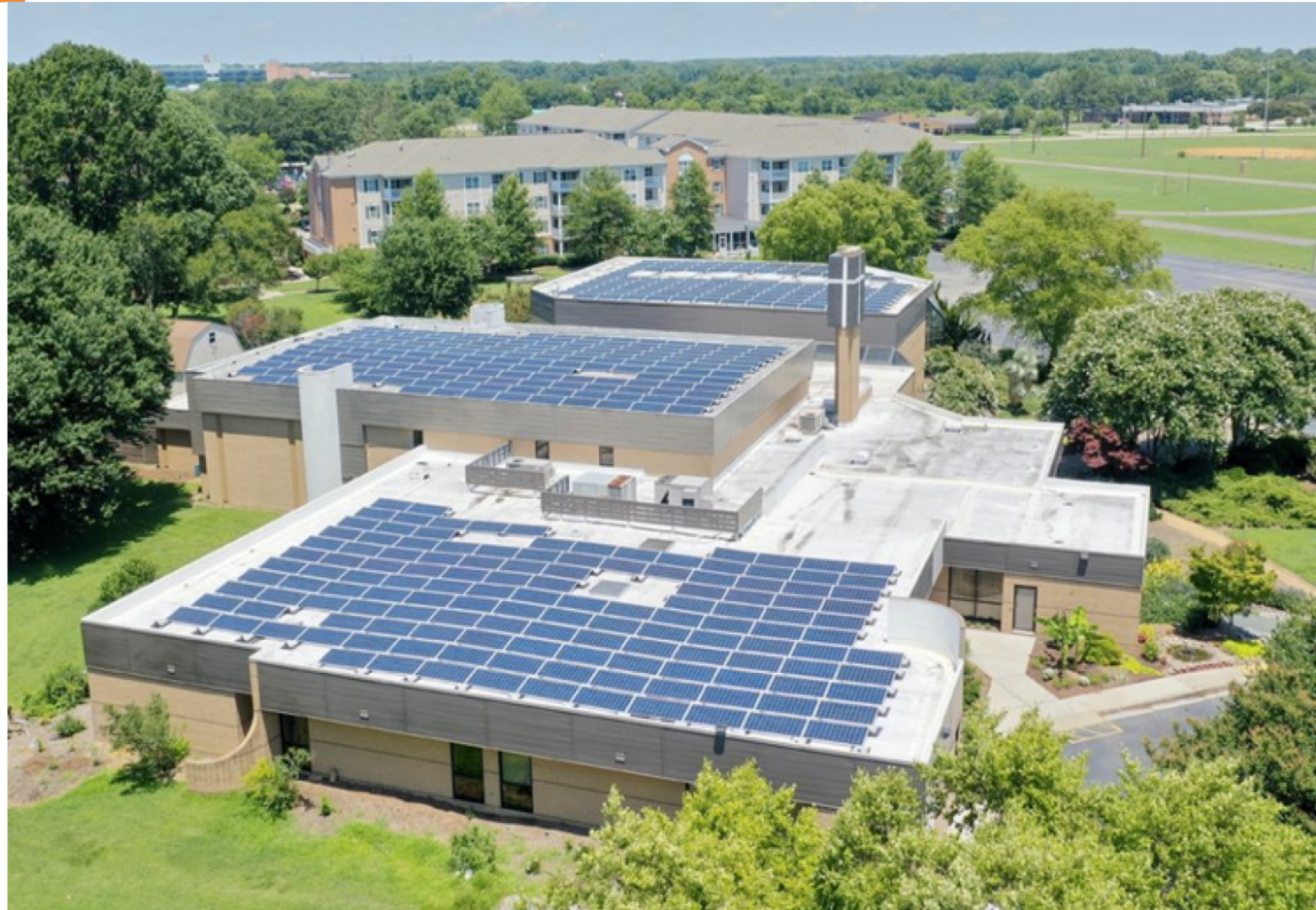
A total of 440 solar panels were installed in June on the church building roof at Immaculate Conception Catholic Church in Hampton, Virginia. (Vy Barto)
